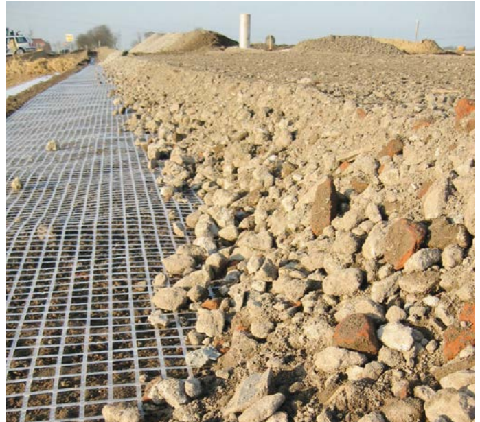
Fig. 19 Crushed base course material over Naue Secugrid® for base stabilisation in access roads
