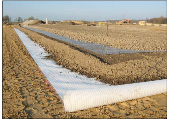
Fig. 8 Base course reinforcement on a very soft subsoil with Naue Combigrig® (bottom) and Naue Secugrid®
